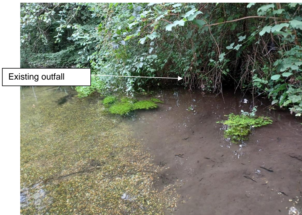
Figure 31 - Existing Outfall Silt Accretion
